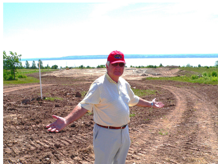
Director of Operations Mike Doyle during construction of Cobble Beach Golf Links near Owen Sound. In background is what is now the par 5 7th hole.
